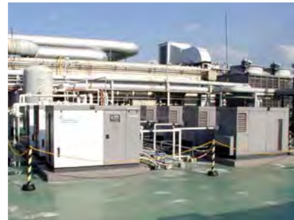
Printing plant: SMS37SD×7
